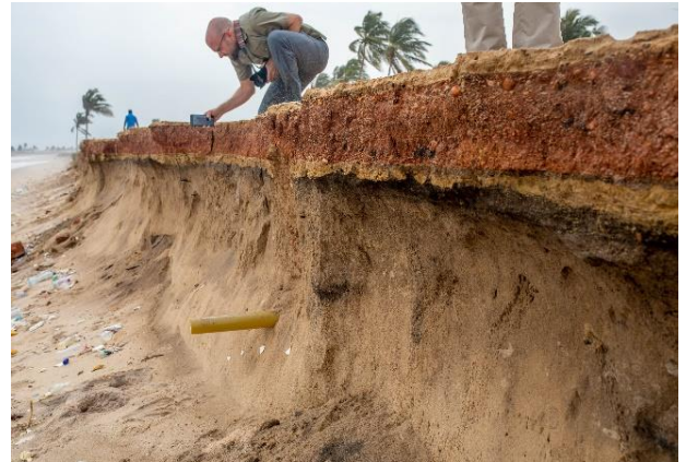
Fig. 15 Erosion observed at the Ada East District of Ghana
